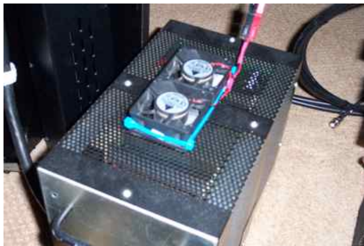
Fan pair in place above the bleeder resistors
