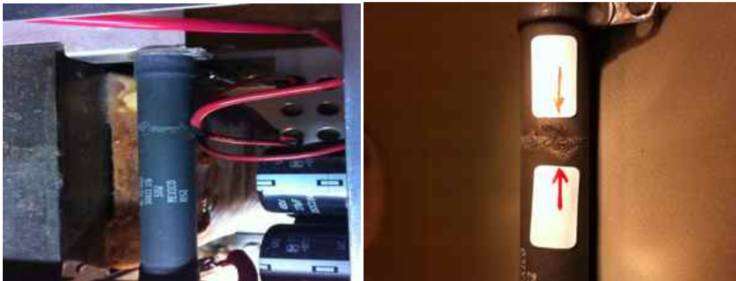
High Voltage Bleeder Resistor Failure
