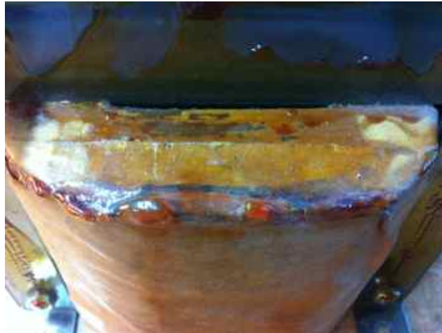
Unusual "ooze" from the transformer's interior
